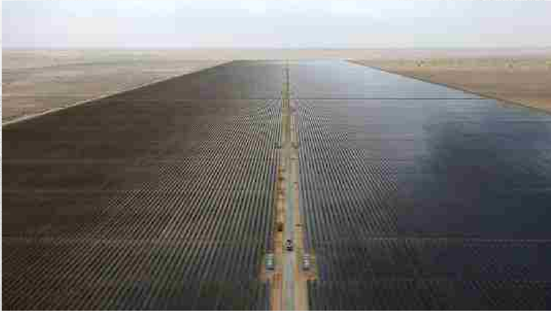
THE MOHAMMED BIN RASHID AL MAKTOUM SOLAR PARK PHASE 5 IN DUBAI. PAWAN SINGH
